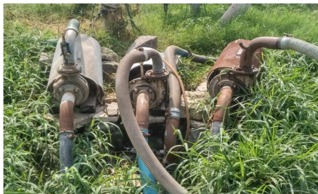
Fig : Pumps at the site
